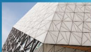
Curtain wall decoration
